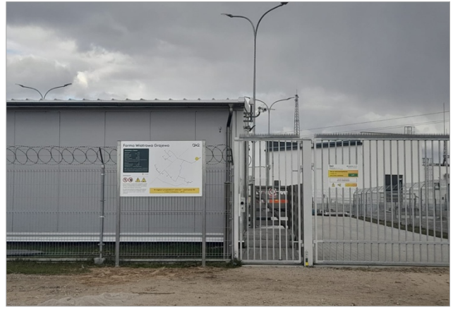
Photo 7.6 Information and warning sign placed in the vicinity of GPO substation
