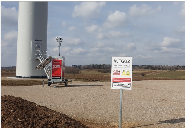
Photo 7.1 Warning sign placed in the vicinity of WTG02
